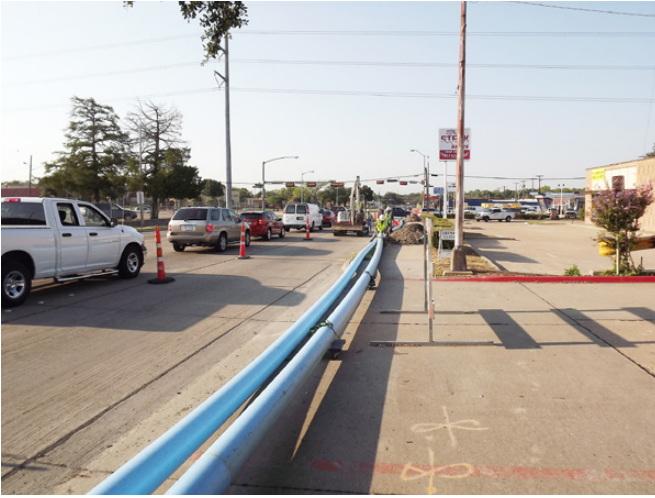
Great value in a contractor being able to upsize a water main while still allowing traffic to flow
