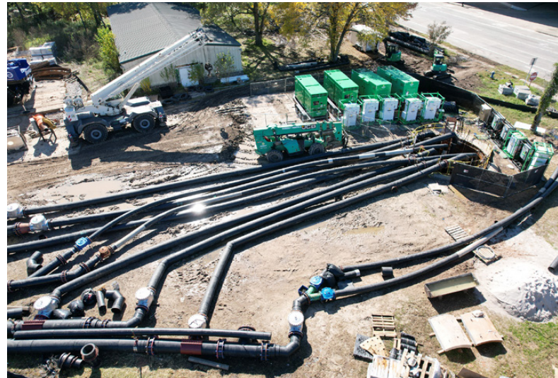
Pumping system worked as designed over the six-month project duration even handling several high wet weather events
