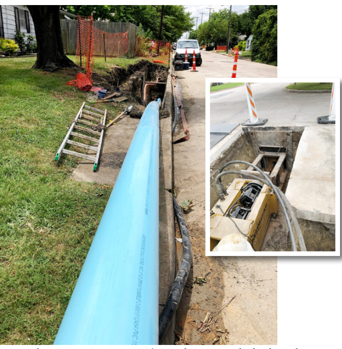
Minimal excavation/restoration. The pipe bursting method reduces digging requirements are reduced as much as 90 percent compared to an open cut “dig and replace” method. The only excavation required is for the pulling machine, insertion pit and accesses to service connections
