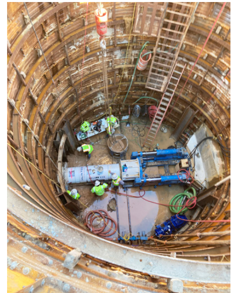
Launching the MTBM on the first 30-inch FRP tunnel drive from MH-T12 to MH-T13 on Talton St.
