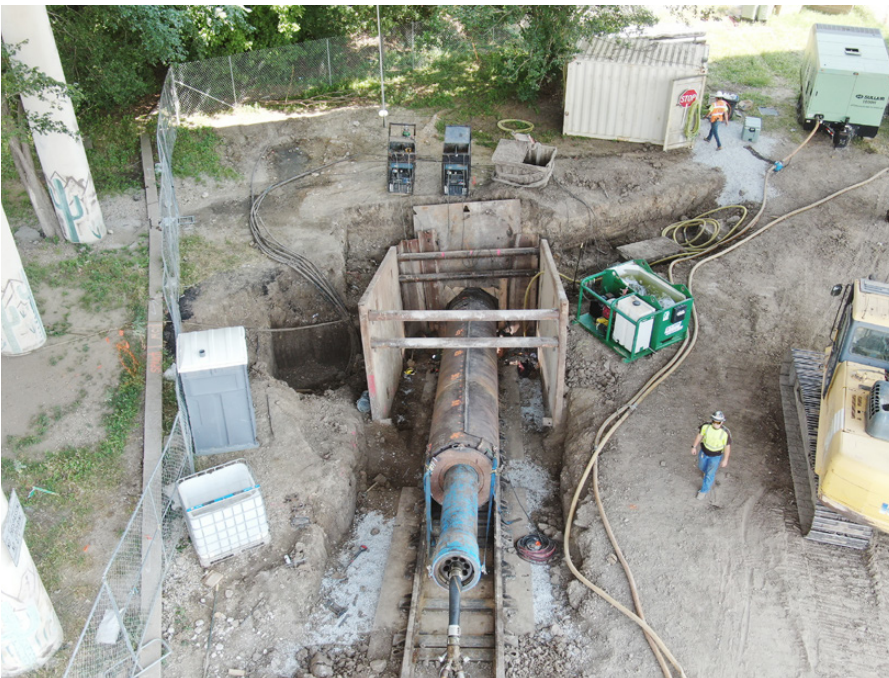
Iowa Trenchless crews installed both Conductor Barrel casings successfully, without incident, using the pneumatic pipe rammer
