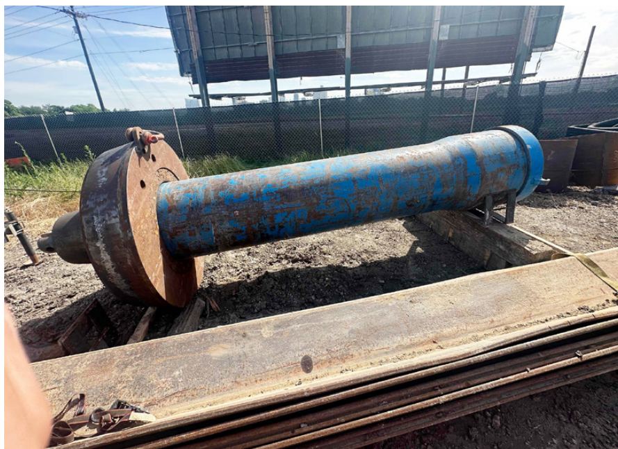
Iowa Trenchless used a Grundroram Pipe Ramming system from TT Technologies to install the Conductor Barrel Casings. Shown: Pipe rammer with ramming gear attached
