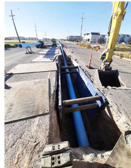
Average slipline pull lengths of 1800 to 2000 feet were achieved by the Contractor
