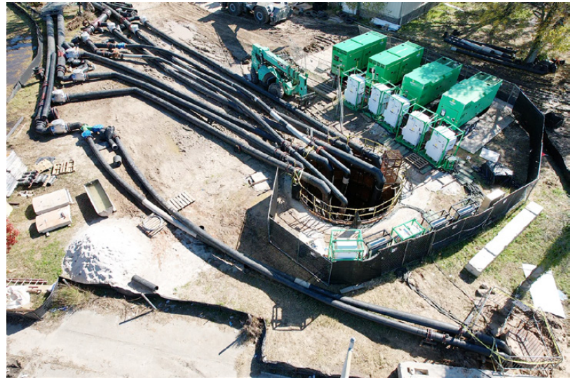
Manhole upstream of the shaft (lower right) was used for two pumps
