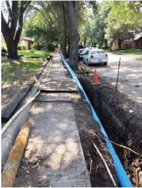
The majority of the insertion pit does not need to be much wider than the pipe itself
