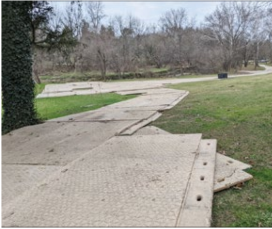
The mats pin together and distribute the weight of equipment over a greater surface area, thereby reducing soil compaction and restoration costs
