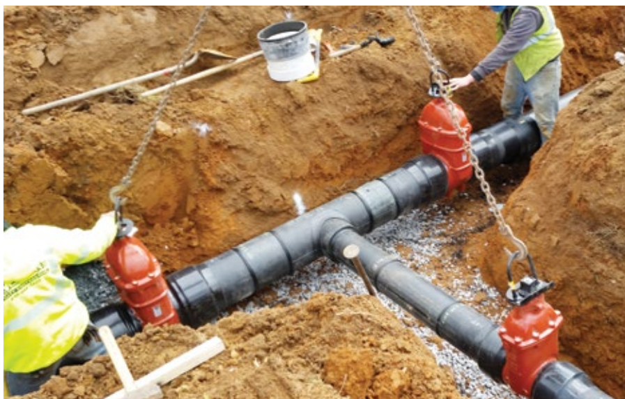
When disinfecting an HDPE potable waterline, it is important that purging applies to distribution mains as well as each service line and service connection.
