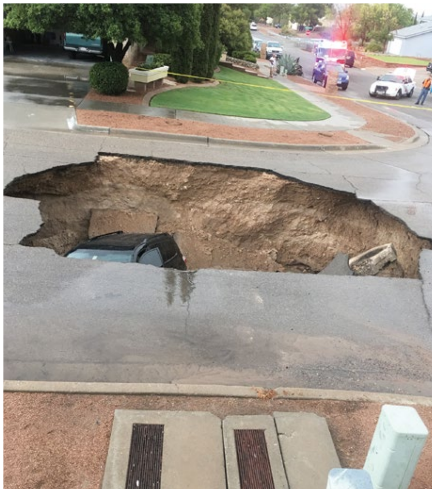
Figure 1 – SUV trapped in the sinkhole (Courtesy of Debra Pazos)
