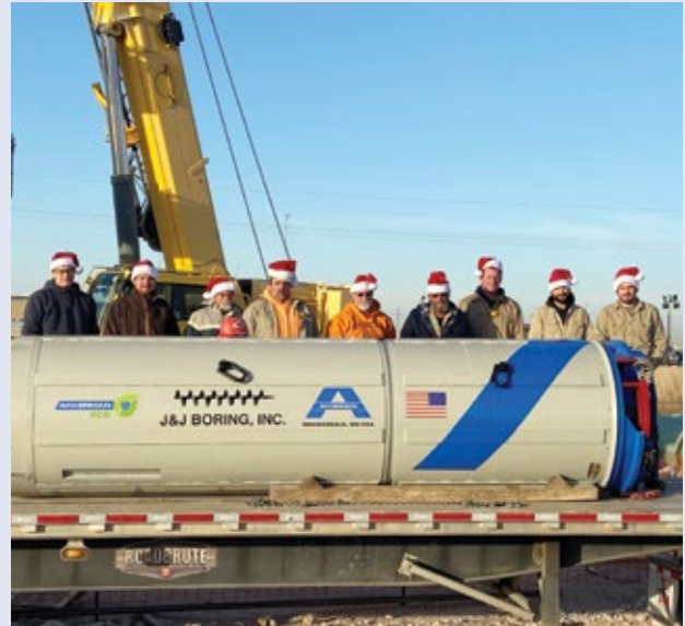
Great Christmas present for the J & J Boring crew to complete tunneling before the holidays!
