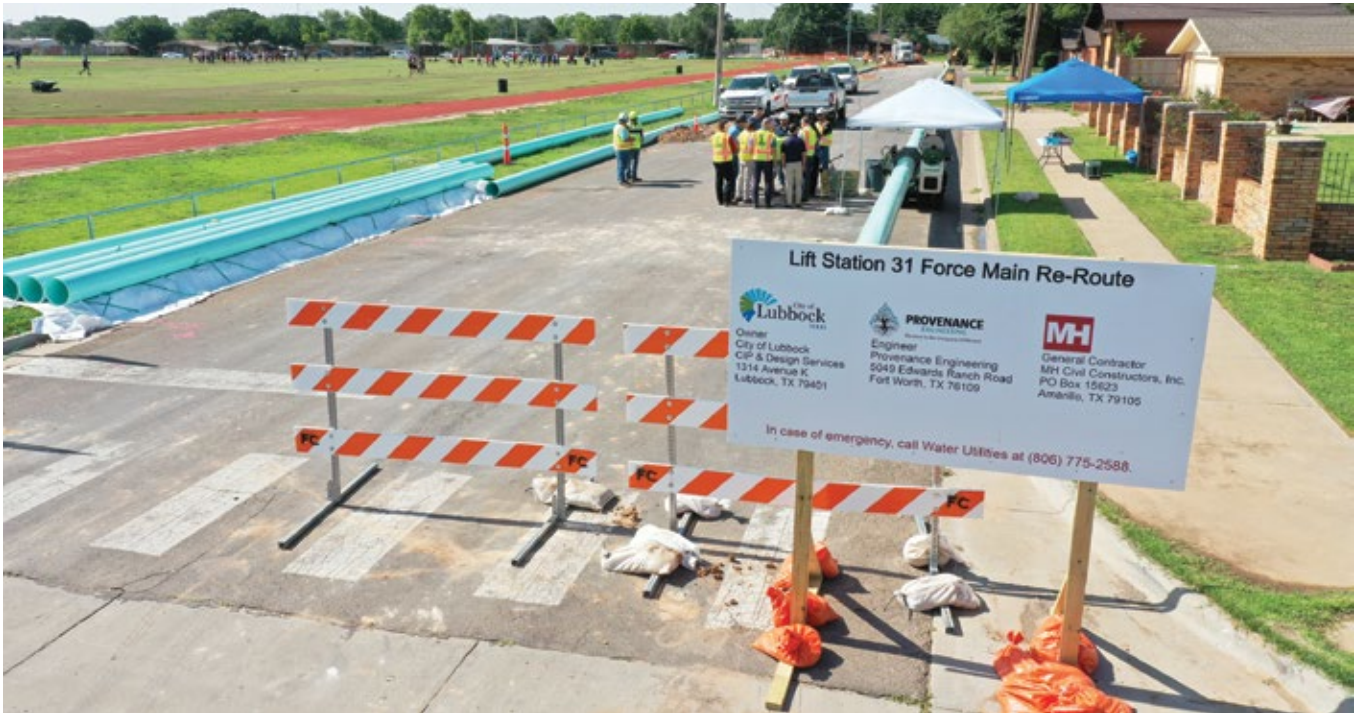
Figure 5. One of Lubbock’s first Fusible PVC pipeline and one of the city’s first full HDD pipe installations.
