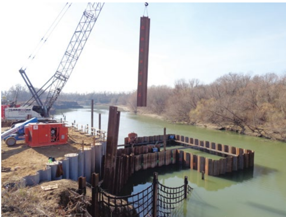
Figure 6. The second microtunnel drive was done as wet retrieval in conjunction with divers
